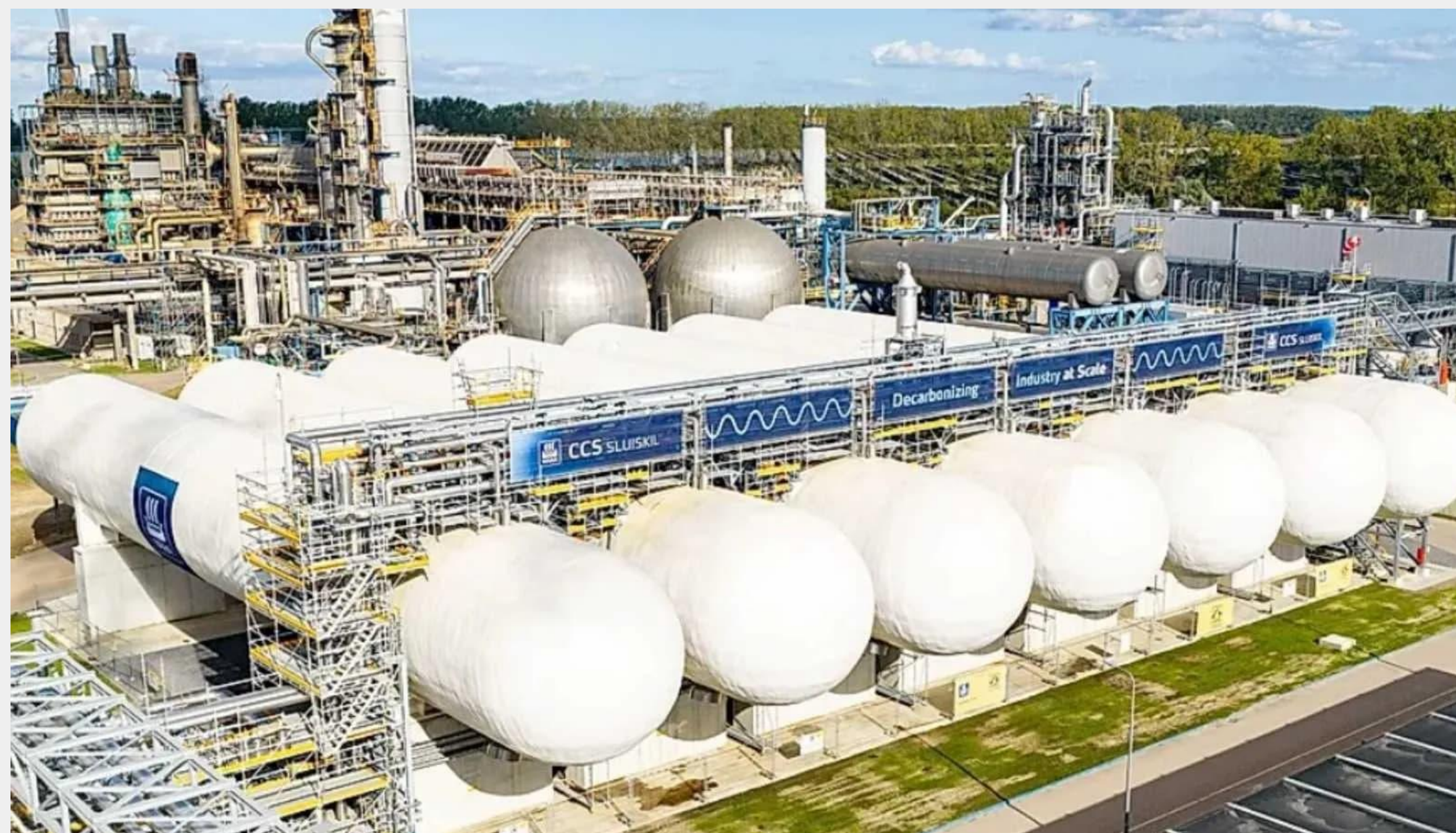
Yara's plant in Sluiskil, the Netherlands
